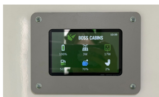
GENERAL INFO AND TANK LEVELS.
